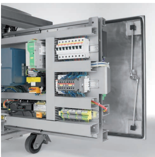
Control hardware arranged for easy maintenance.
